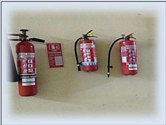
Fire extinguishers mounted at the walls
