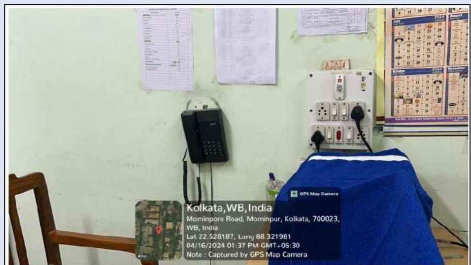
INTERCOM facilities in the college Office and Common Staff Room
